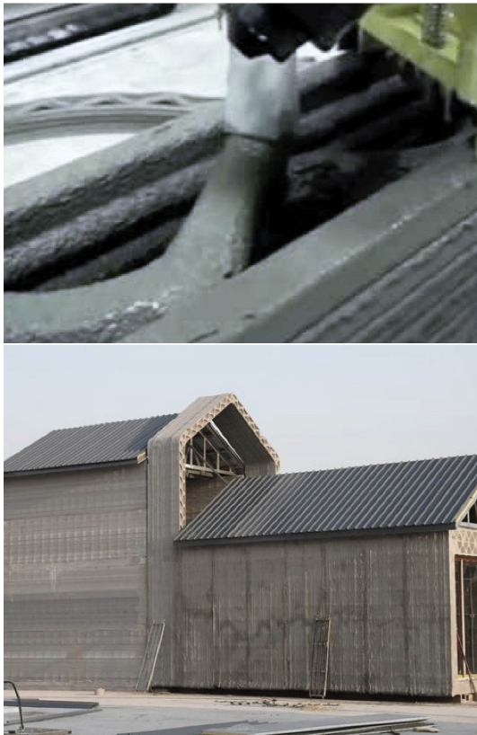
Figure 3. (Top) Contour Crafting, with layers of approximately 5 cm. (Bottom) House printed and assembled by WinSun.
