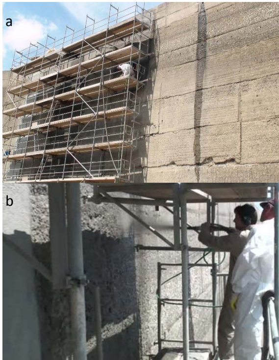
Figure 7. a) Condition of the upper water reservoir of the pumping hydraulic power station Hohenwarte II in Thüringen, Germany before repair, b) spray-application of highly ductile, cement-based composite containing SAP as repair material
