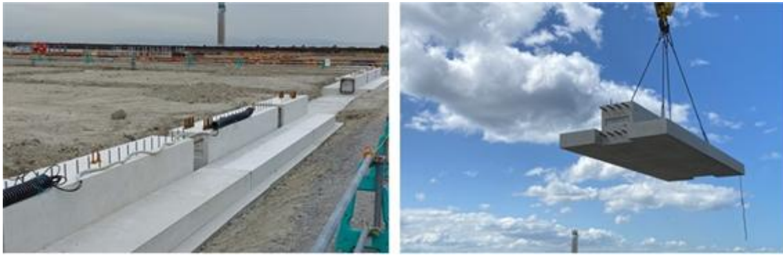
Figure 9. Application of CCUS pre-cast concrete elements at WASSE (the nickname for the event field), Expo 2025 Osaka, Kansai, Japan (Original photographs).
