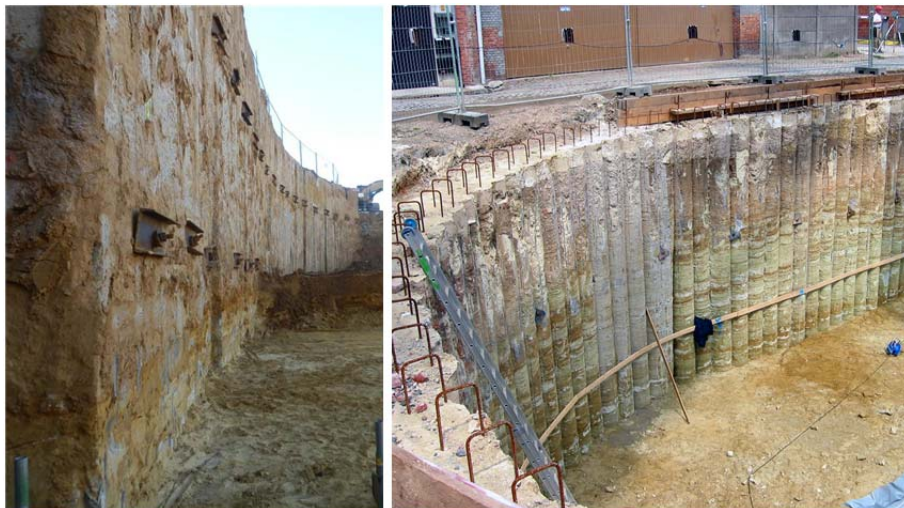
Figure 2. Soil mix retaining walls within the framework of excavation works in Belgium: soil mix walls built with CSM-panels (left) and with the C-mix shaft system of CVR nv (right) .
