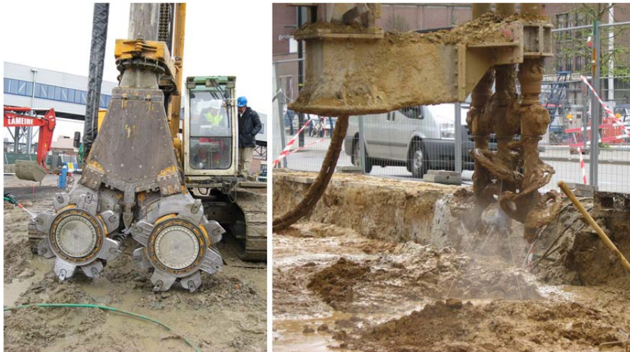
Figure 1. Illustration of typical deep mixing equipment in action on Belgian construction sites: Cutter Soil Mix (CSM) system of Bauer (left) and triple shaft configuration TSM system of Smet F&C (right).
