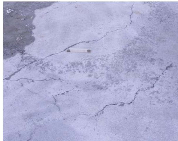
Figure 1. Plastic shrinkage cracks appearing on the concrete surface few hours after placement. Photo courtesy of Dr. Andreas Leemann, Empa.
