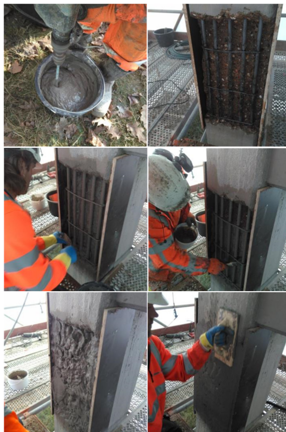
Figure 5. On site structural repair of damaged steel reinforced concrete column with bacteria-based self-healing repair mortar.
