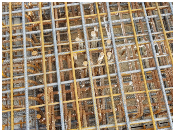
Figure 4. Picture of a finely meshed reinforcement network for watertight concrete constructions impeding easy casting of concrete.
