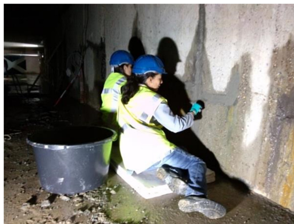
Figure 6. Manual repair of actively leaking cracked concrete basement walls using bacteria-based self-healing repair mortar.
