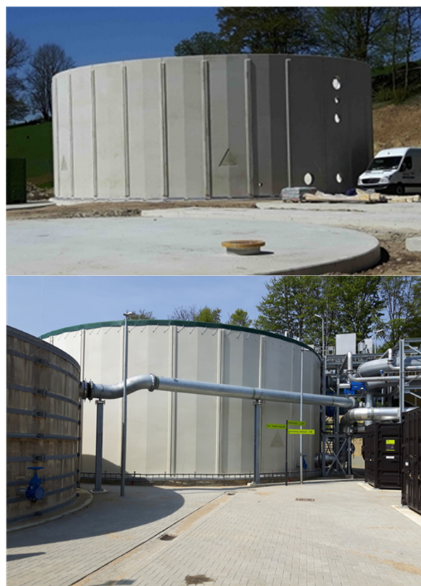
Figure 7. Prefabricated wastewater treatment tank under construction (top image) and in service (bottom image). Prefab elements bearing the triangular logo contain self-healing agent while the other, reference elements, do not.
