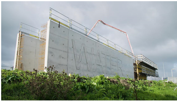
Figure 8. Full scale demonstrator in situ cast self-healing concrete water reservoir, Hoogvliet, The Netherlands.
